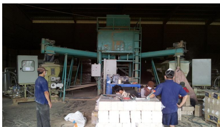
FIGURE 10: A SAWDUST BRIQUETTE PRODUCING LINE IN VIET PHAT BIO CORP
