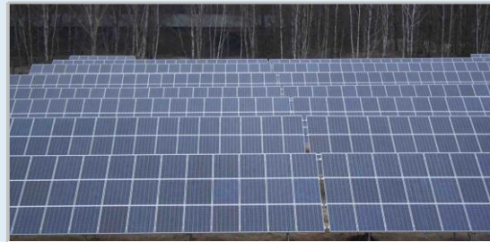
Germany - "Schierling", 0.5 MW 2013
