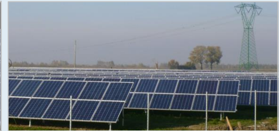
Germany - "Schlieben Berga", 0.3 MW 2013
