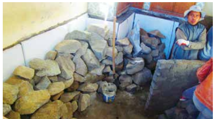
Figure 5. Pebble bed thermal energy storage at Kurja guest house in Leh
