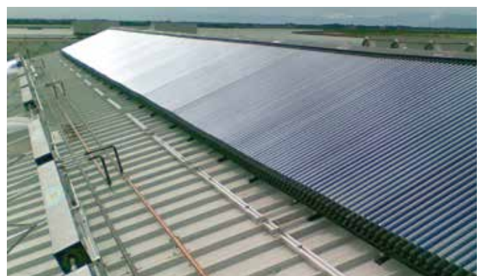
The installed solar heat system
