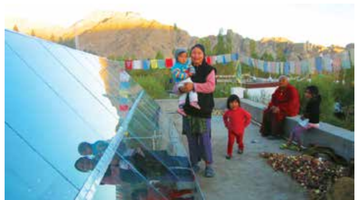
Figure 4: A demonstration solar air heating system installed on the roof of a house in Leh
