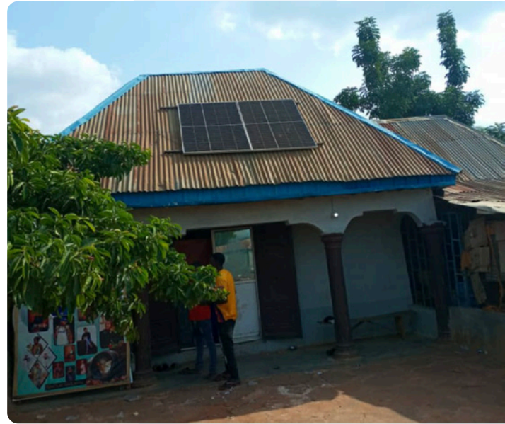
Figure 4. LiteDey System powering a clothes retail shop (Source: CREEDS)
