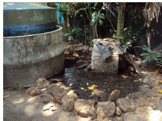
Figure 30: Accumulation of the effluent in the surroundings of the plant.
