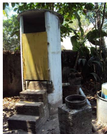
Figure 31: BIOTECH latrines having a difficult access.
