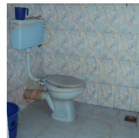
Figure 15: Toilet connected to plant 2 with a 4L toilet flush.
