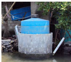
Figure 9: 2m 3 toilet linked plant in Kumbalangi.
