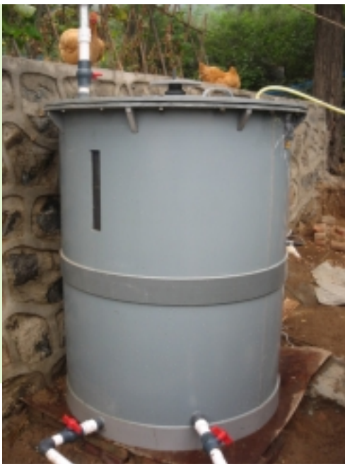
Figure 3: PVC Above Ground Biogas Digestion Tank
