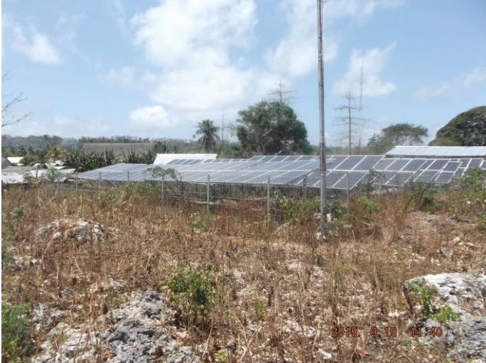
Figure 19 – A 50 kWp capacity of Solar Power Plant (PLTS) in Larat Island
