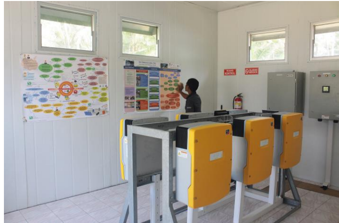
Figure 26 – Posters of Solar Power Plant (PLTS) troubleshooting to help the operator
