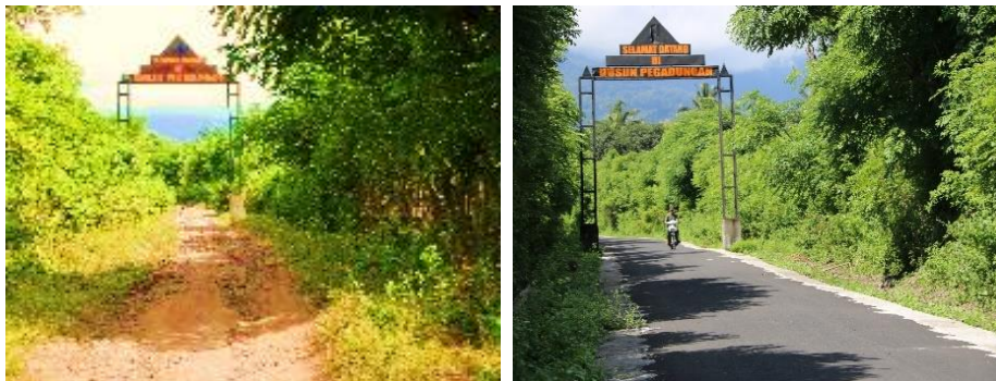
Access road to Hamlet of Pegadungan before and after the paving work with hotmix asphalt
