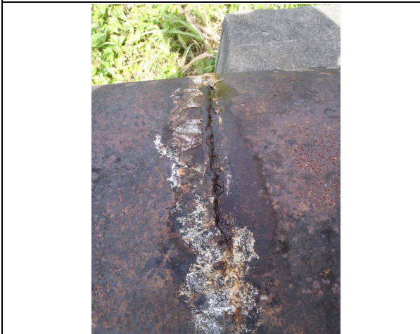
Photo 3: Corrosion at penstock in Wonorejo, Oct 10
