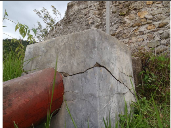
Photo 18: Anchor block broken due to earthquake, Sungai Kalu Oct 10
