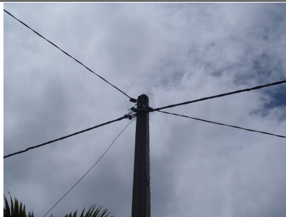
Photo 21: Concrete pole with well fixed cables in Sungai Kalu, Oct 10
