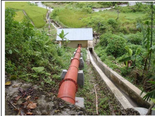
Photo 17: Penstock in Limau Limau, Oct 10
