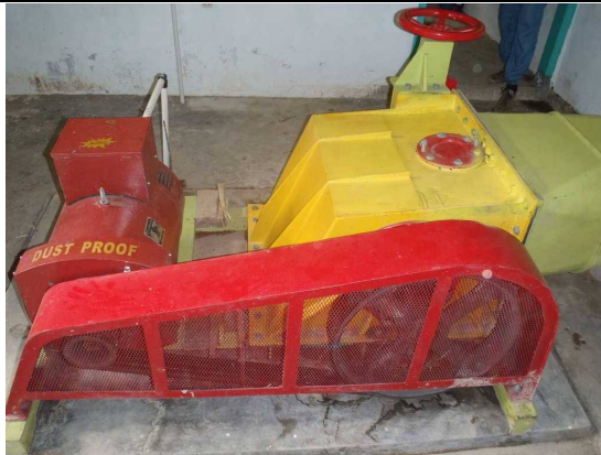
Photo 19: Properly operating turbine with generator and protection on belt, Oct 20
