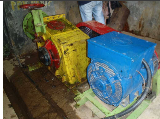
Photo 20: Turbine with leakage and too much grease in Sungai Kalu, Oct 10
