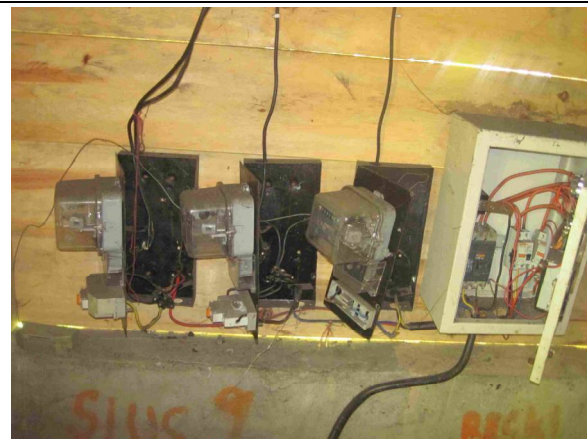
Photo 22: Not well maintained electrical installations in powerhouse in Minangga, Oct 10
