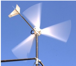
Roof-mounted urban wind turbine charges a 12 volt battery and runs various 12 volt appliances within the building on which it is installed
