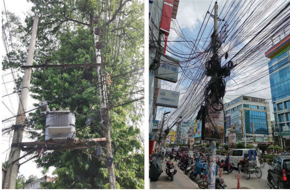
Tangled power lines. Poor power distribution networks can affect supply, as in Dhaka and Khulna, Bangladesh (photos by the author).
