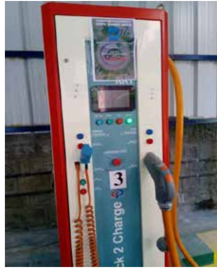
Figure 2.5: EVSE installed at BESCOM [44]
