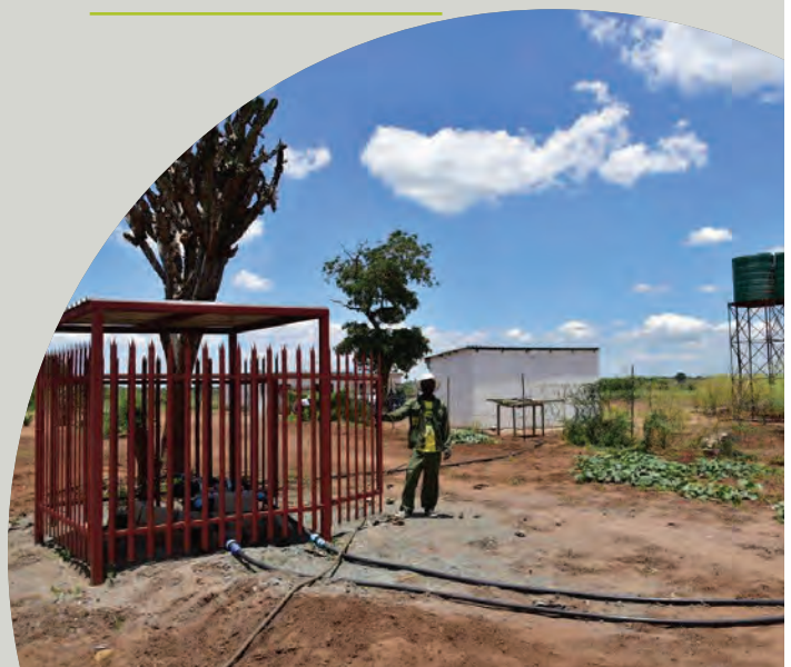
Phepisa site showing water storage, pump and generator room
