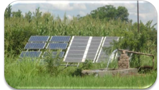
Solar Irrigation System in India, GIZ/ Pullenkav
