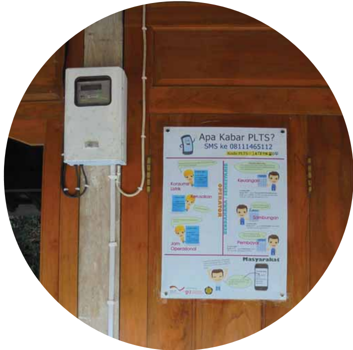
Contact details to Energi Desa are displayed on posters generally mounted at the community centre or powerhouse. A more simple contact number “2000” is now used in the system.
