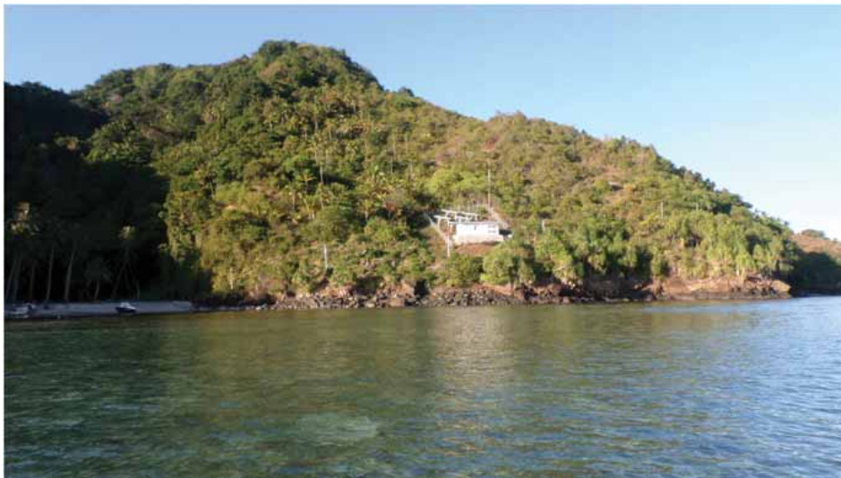
This PVVP installation on a small remote rocky island demonstrates the installation challenges faced by contractors.
