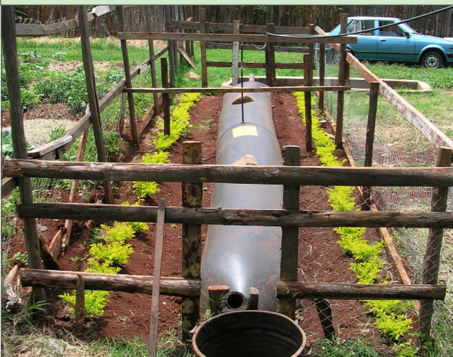
Figure 60: Biogas Generator by Pioneer. Source: © SuSanA Secretariat
