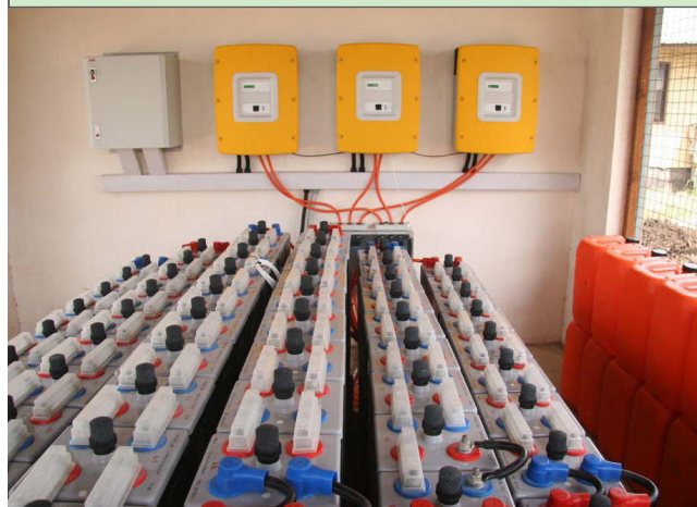
Figure 53: Flooded deep discharge lead-acid battery bank feeding three SMA Sunny Island inverter/chargers. Image Source: © DreamPower Solar.
