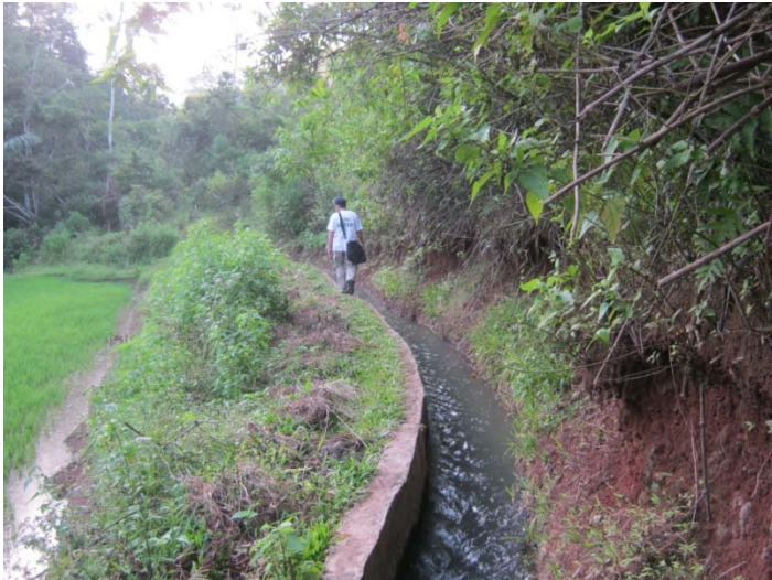
Exhibit 2.9b: Only One Side of the Channel is strengthened with Concrete, Saluburonan, Non-TSU site
