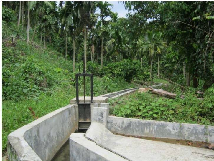
Exhibit 2.9a: Both Sides of Channel are Sthrengthened with Concrete, Alur Kejrun, TSU site
