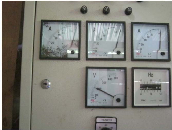
Exhibit 2.8: Damaged control panel, 2 years after commencement of operation
