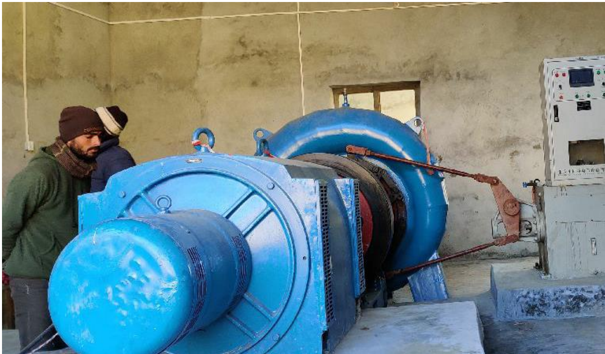
Figure 2-3: Turbine Generator Set of 200 kW Giri Khola MHP
