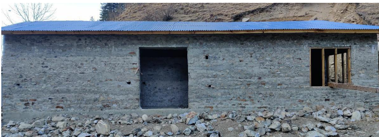
Figure 2-1: Building on place of Powerhouse of Chukeni MHP (Probably Control Panel Building)
