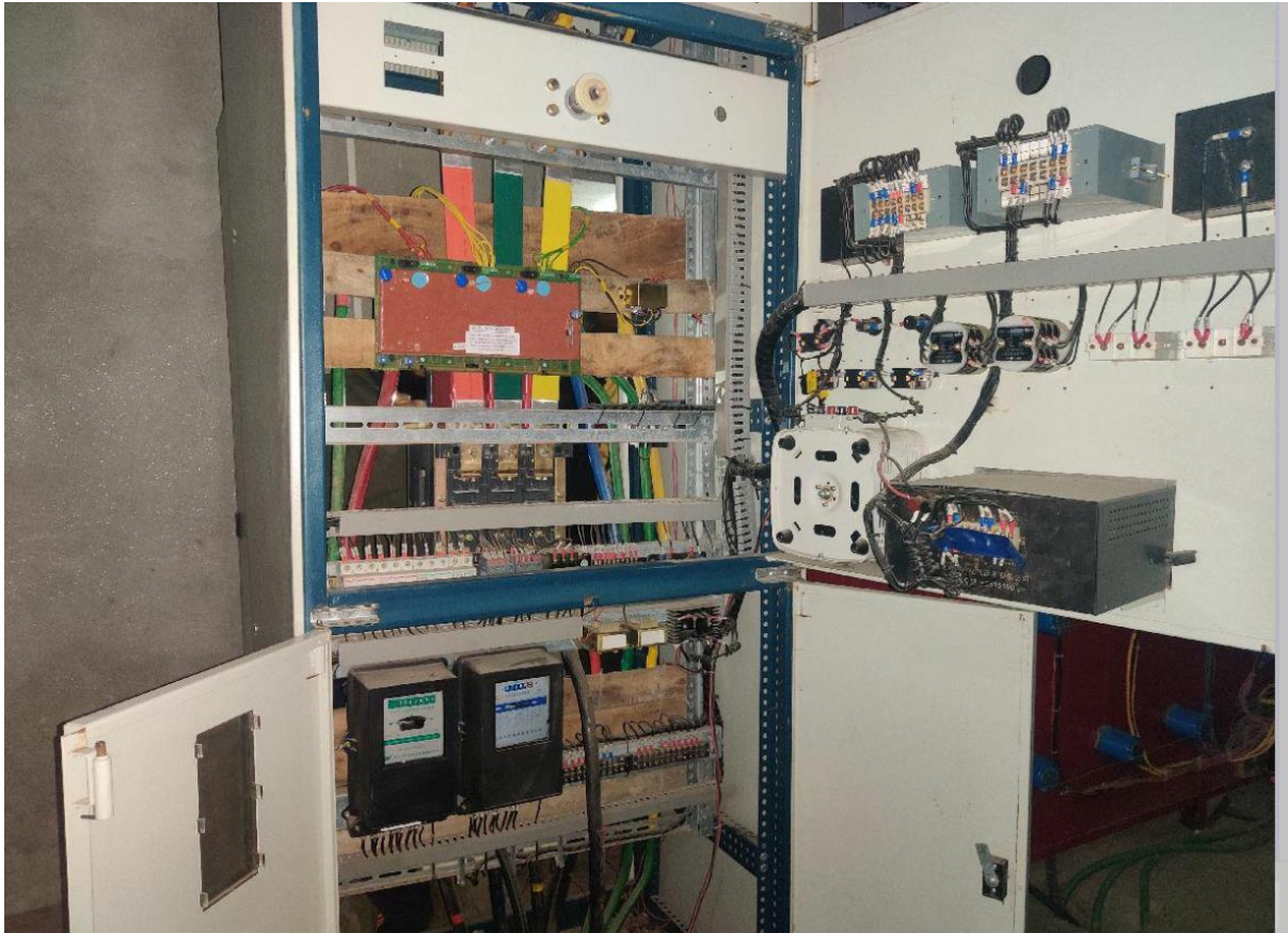
Figure 2-4: Existing Metering Panel of Thinke Badh
