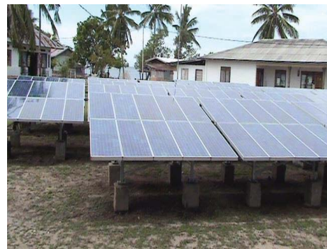
Photo 4: Centralised PV System, Ponelo Island, Gorontalo, Sulawesi
