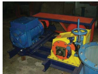
Photo 16: Cross-flow turbine and generator, Bandung, W. Java
