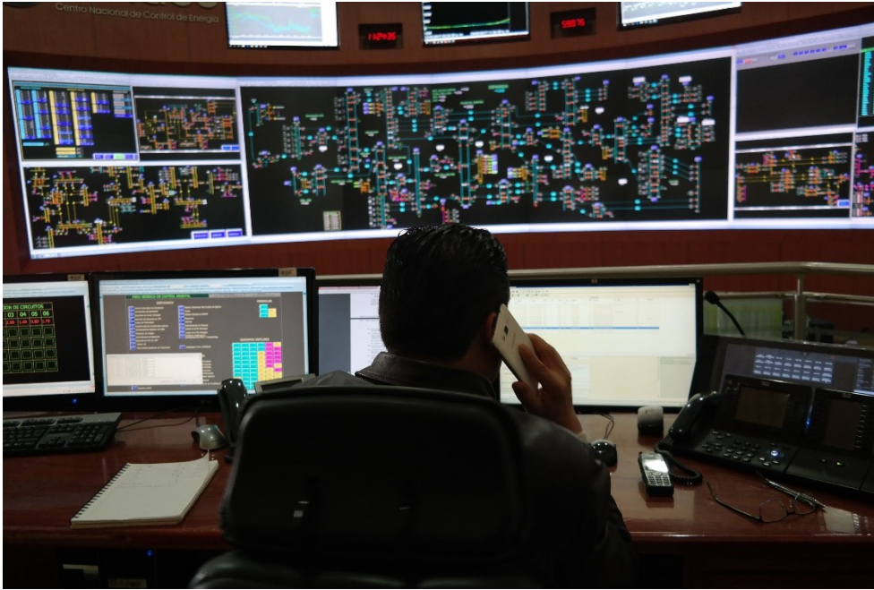
Figure 19: Typical control room of a TSO. Source: energy & meteo systems
