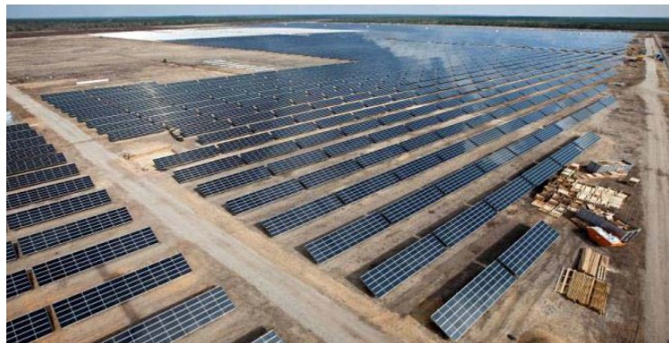
52,79 MW free-field installation, Lieberose (Brandenburg)
