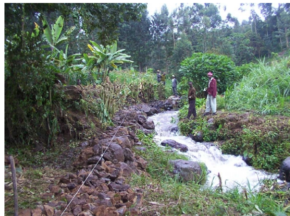
A few hours later, a stone platform has been constructed to support the pipe.
