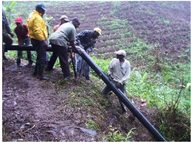
Since PVC is quite rigid, 45° elbows joints were cemented in at two points to enable the penstock to follow the shortest path to the turbine house.
