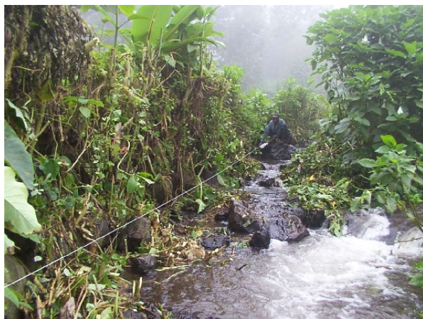
The penstock level is marked out with string up to the proposed intake position.
