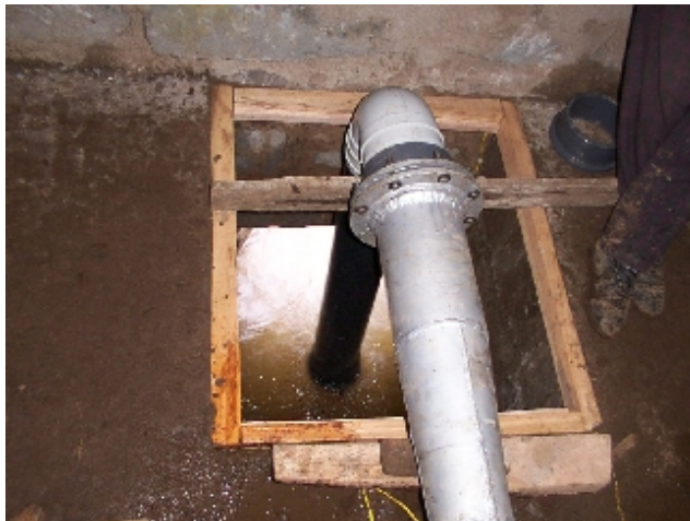
A draft tube increases the head by 1m whilst ensuring that the turbine remains above flood level.
