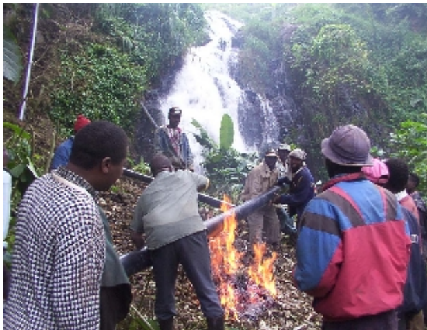
Small bends were made by heating sections and then shaping around a former. Embers rather than flames (as above) should be used to avoid the risk of melting the pipe completely.
