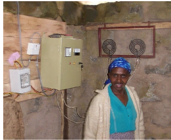
Two 1.8kW cooking rings have been used as a ballast load. An RCD (left) improves consumer safety by minimising the risk of dangerous electric shocks.
