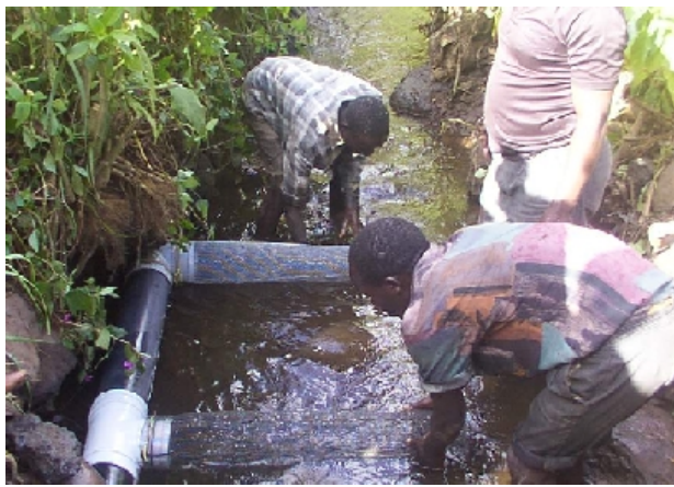
Galvanised wire mesh prevents debris from entering the penstock at the intake
