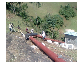
Penstock and power house
