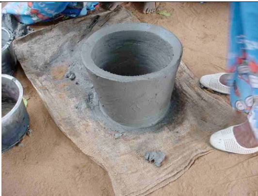
flatten the top with an inclination sloping inside to help gases escape from the firebox
