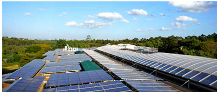
Figure 4.5: PV roof integration, UNEP building in Nairobi, Kenya
