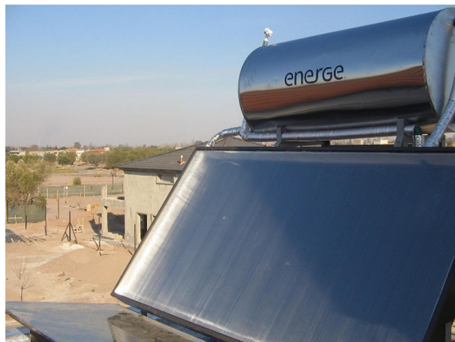
Figure 4.8: Roof mounted flat plate collector with close-coupled thermosiphon heat storage
