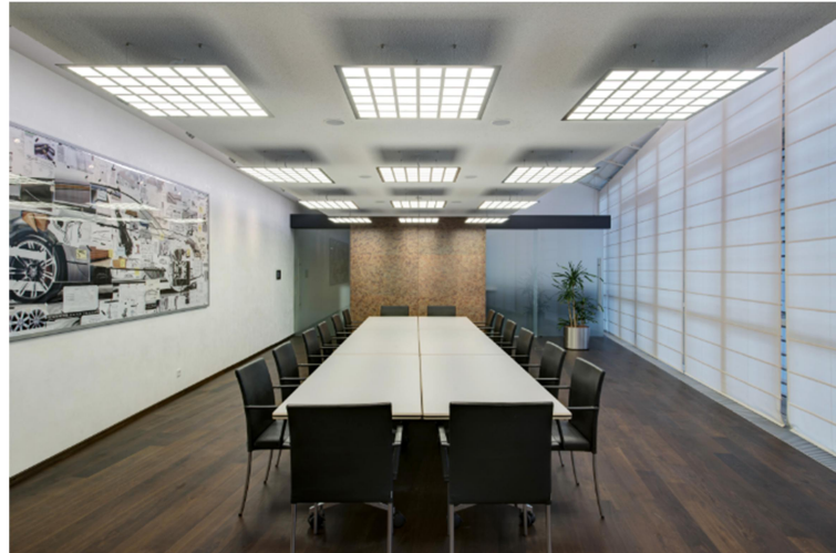
Figure 3.57: OLED luminaires suspended from ceiling, Audi visitor's centre, Ingolstadt, Germany (photo: Mueller, H.)
