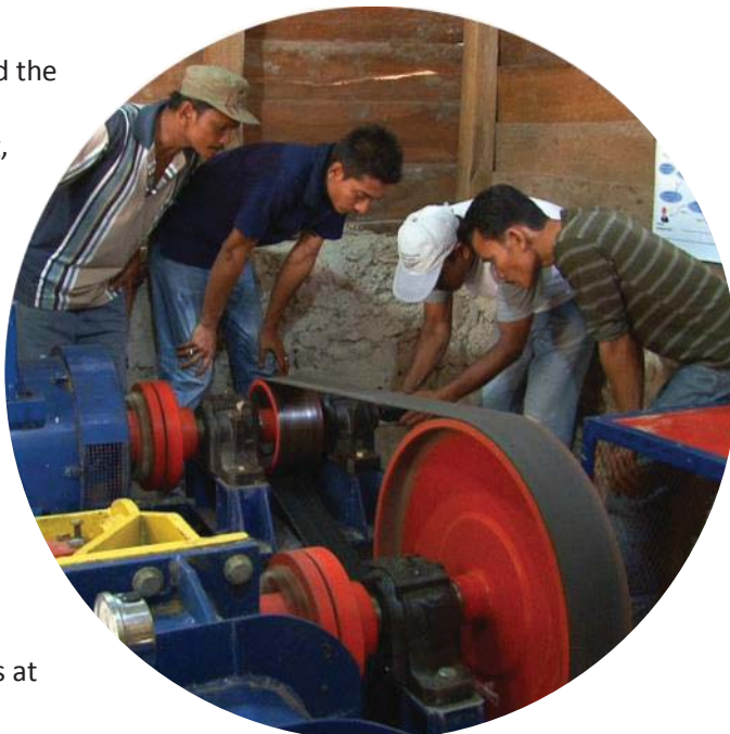
Operator gets a first-hand experience on how to operate and check the turbine.
