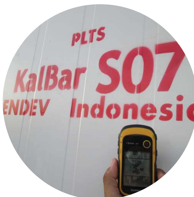
EnDev ID allocates a unique identification number to each site. This number is also spray painted to the powerhouse.
