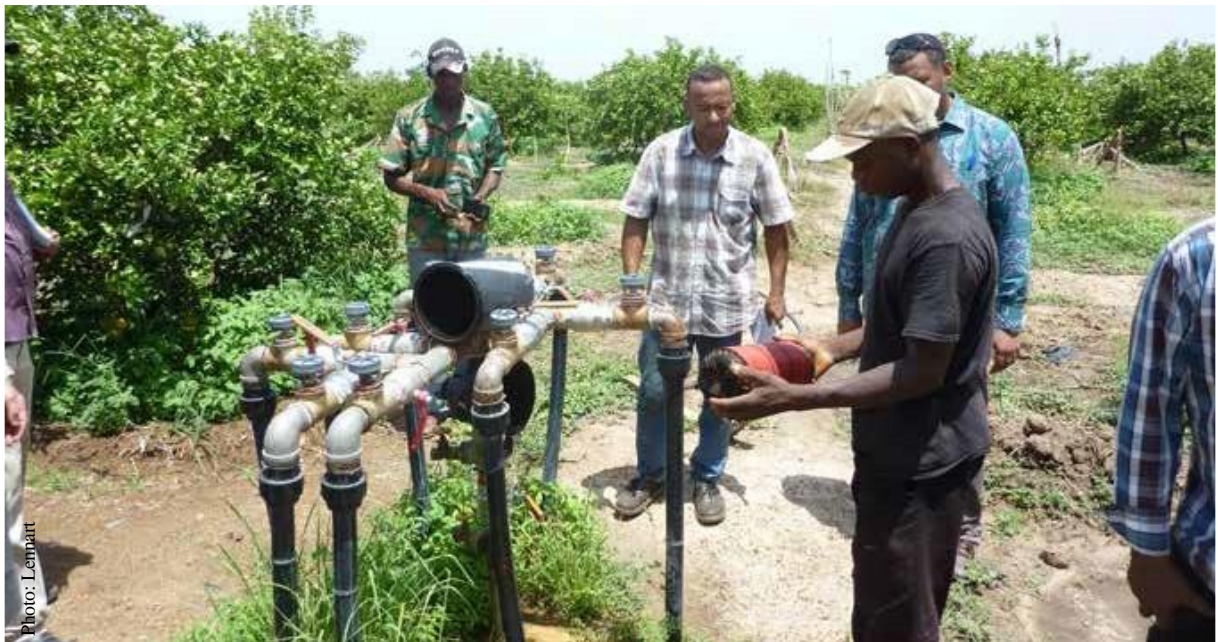
Irrigation head with a disc filter and multiple valves that guide the water to different sections of the irrigation system (Source: Lennart Woltering).
