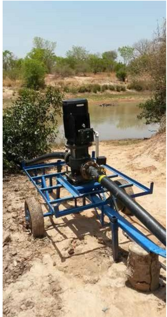
Surface pump on a mobile structure (Source: Lennart Woltering)
