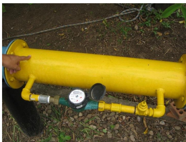
Water metering of source water with a low-cost proportional water meter
