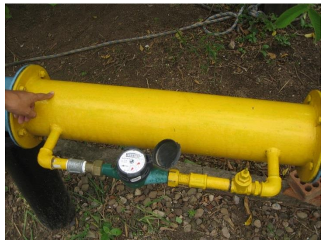
Water metering of source water with a low-cost proportional water meter
