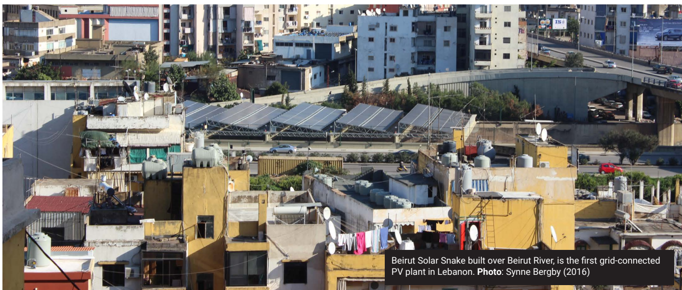
Solar PV in Burj Hammoud, Beirut, part of community upgrading project by PCPM, UN-Habitat, the municipality, and LCEC. Photo: LCEC (2020).
