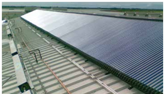
The installed solar heat system
