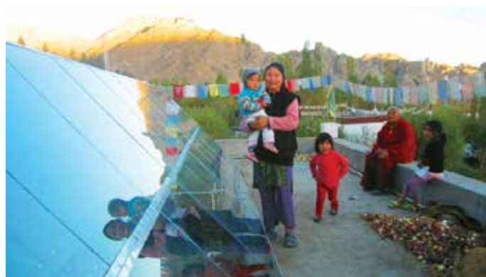
Figure 4: A demonstration solar air heating system installed on the roof of a house in Leh
