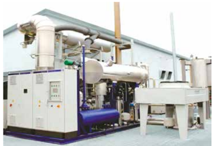
Figure-1 ORC system in Groß-Gerau
