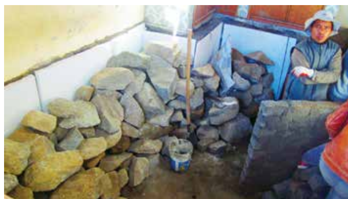
Figure 5. Pebble bed thermal energy storage at Kurja guest house in Leh
