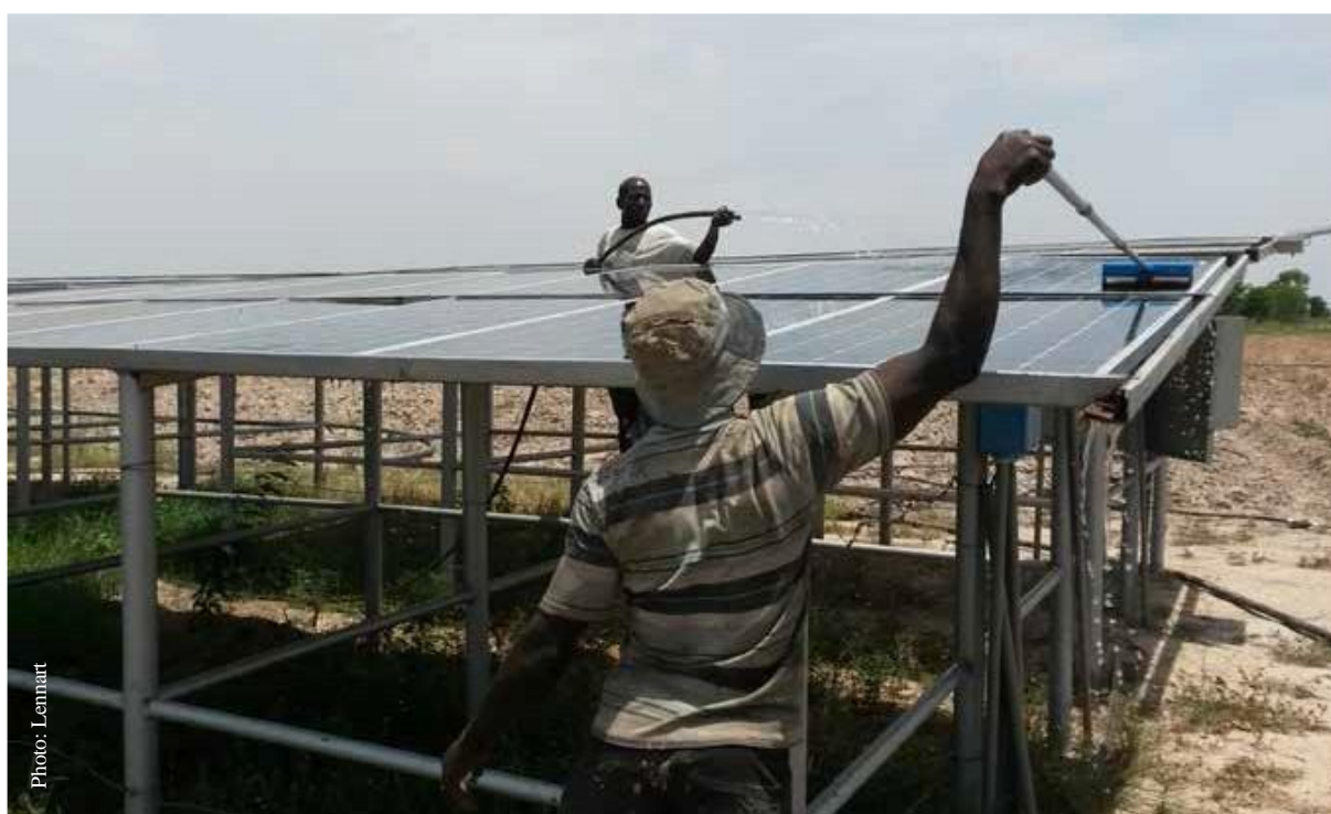
Cleaning of solar panels in Ghana as a routine maintenance activity (Source: Lennart Woltering)
