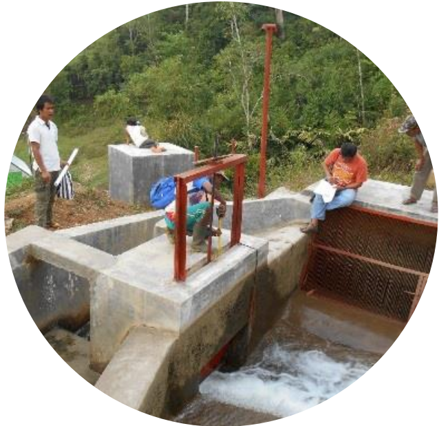
Assessing the civil work of a micro hydro power requires thoroughness and carefulness. (Source: EnDev ID, GIZ)
