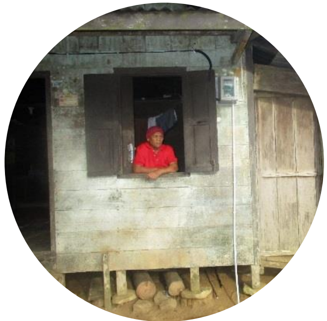
Proper household installation with appropriate grounding and energy limiter protected from the weather. (Source: EnDev ID, GIZ)
