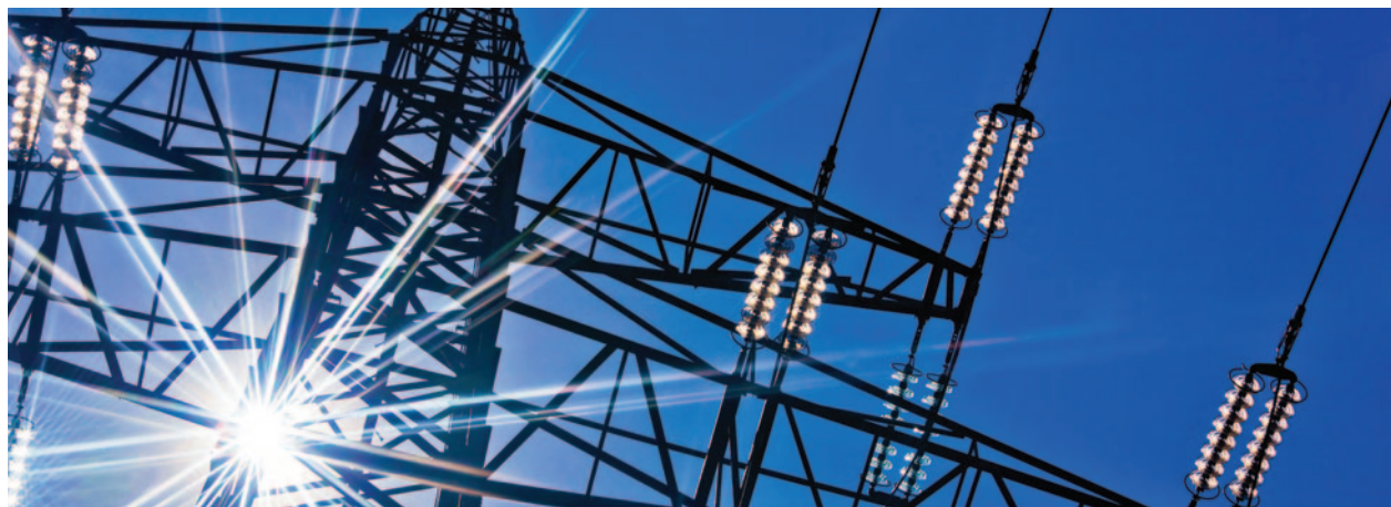
Electricity pylon. © Lisa S
