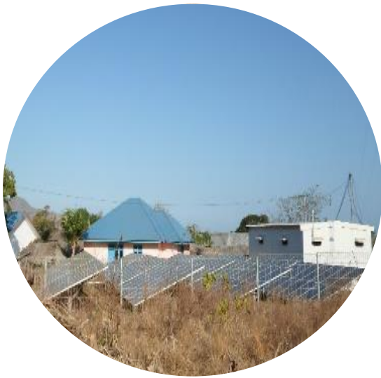
Figure 4 The 15 kWp PV mini-grid in Wetar serving 157 households (MalS11)
