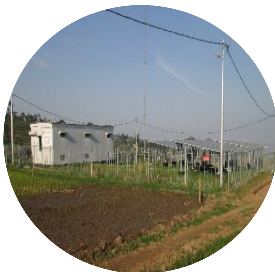
Figure 3 The 15 kWp PV mini-grid in Tegal serving 75 households (JaTengS06)
