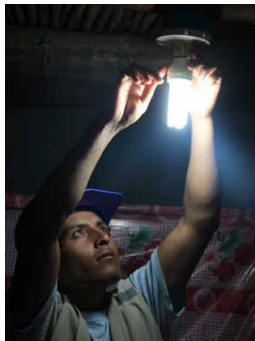
Tito, a young local technician, in the process of final installation and of a safe electrical
