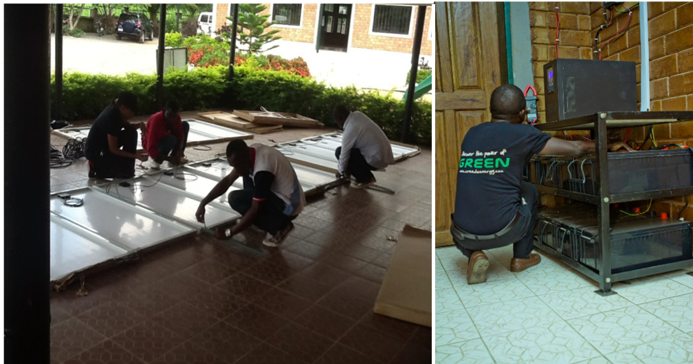
Figure 4.43: PV array and battery checks
