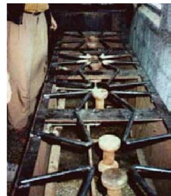
Figure 3.173: Cooking range operating with biogas.
