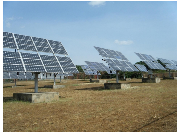
Figure 3.29: Field of solar panel arrays
