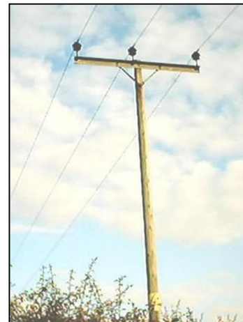
Figure 4.8: Europe, the United States and other areas utilise a three-wire three-phase system
