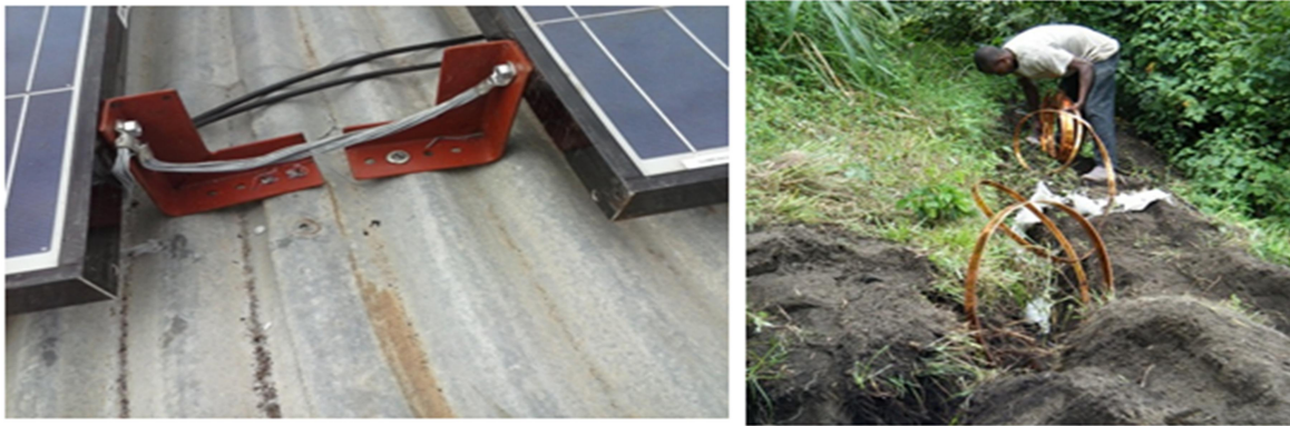
Figure 3.87: Equipotential bonding of module frames (left), laying a ground termination conductor (right)
