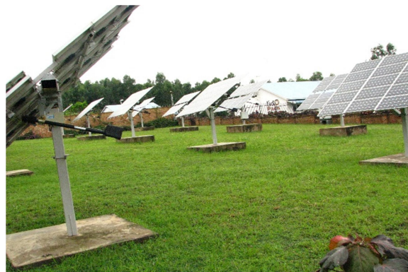
Figure 3.44: Tracking systems mounted on poles
