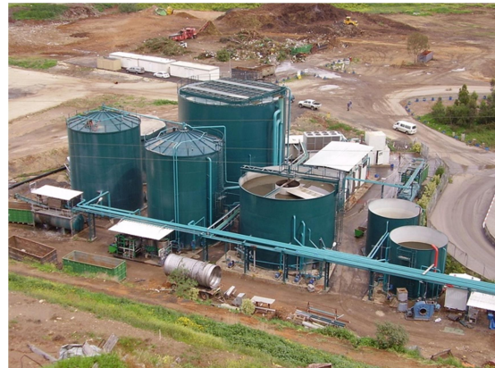
Figure 3.170: Industrial-scale biogas plant in Germany – Courtesy: Wikipedia
