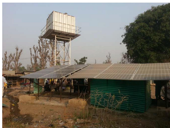
Figure 5.5: Solar array in Roguwa community
