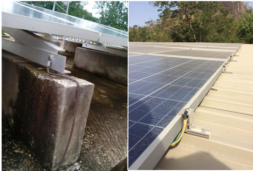
Figure 3.90: Grounded solar array: Ground mounted (left) and roof mounted (right)
