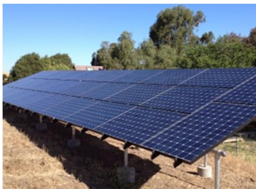
Figure 3.43: Ground-mounted solar PV array – Courtesy: Melissa Van Hoorne, http://blog.solarmicronics.co (accessed Jan. 28, 2016.)
