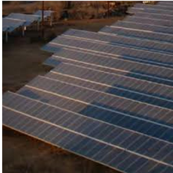
Figure 3.102: Shadow caused by poorly spaced solar PV modules
