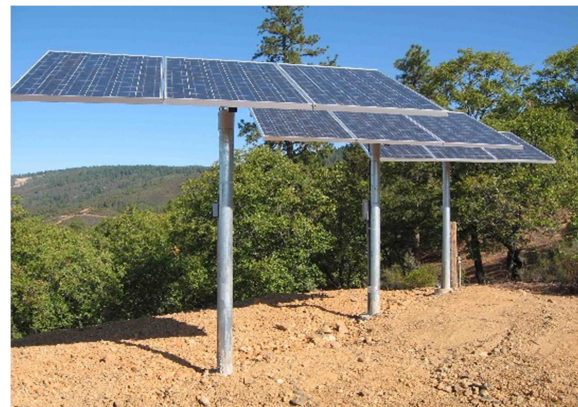
Figure 3.42: Pole-mounted PV array – Courtesy: Accutrack Solar Systems, www.accutrack.com
