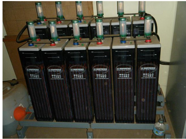
Figure 3.56: 2 V/800 Ah to form a 24 V/800 Ah battery bank
