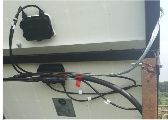
Figure 3.81: Shielded cable connecting inverter, charge controller and ground
