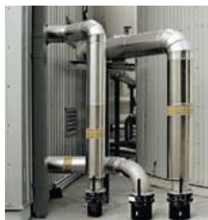
Piping: many years of experience in industrial plant construction
