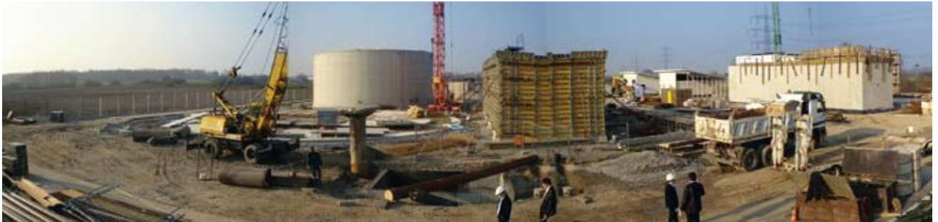
First stage of completion of a biomass power plant consisting of two identical systems
