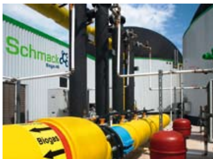
Bio natural gas to be fed into the natural gas network
