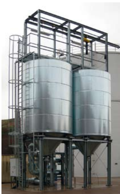
1-chamber gas treatment module
