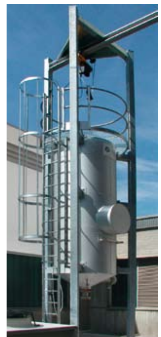
2-chamber gas treatment module
