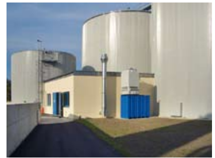
Schwarting biogas plant in Klein Eichholz
