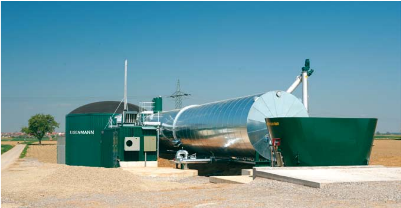
EISENMANN biogas plant with horizontal main fermenter
