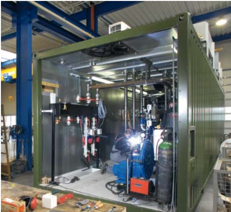
High-technology from Germany: Most equipment is installed in compact containers
