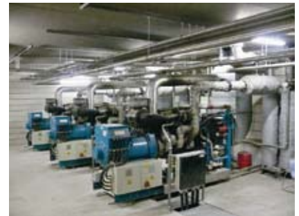
Cogeneration unit inside a building
