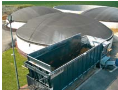
Vielfraß feeding system and Biogene gas storage facility
