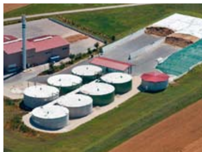
Polystyrene-insulated concrete digester featuring the NQ-150 and SUMA giantmix as well as the NQ-feeding and heating systems (14 independent circles).
