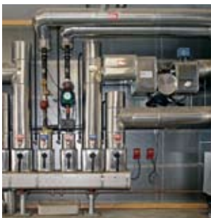
Heat pipelines in a cogeneration unit
