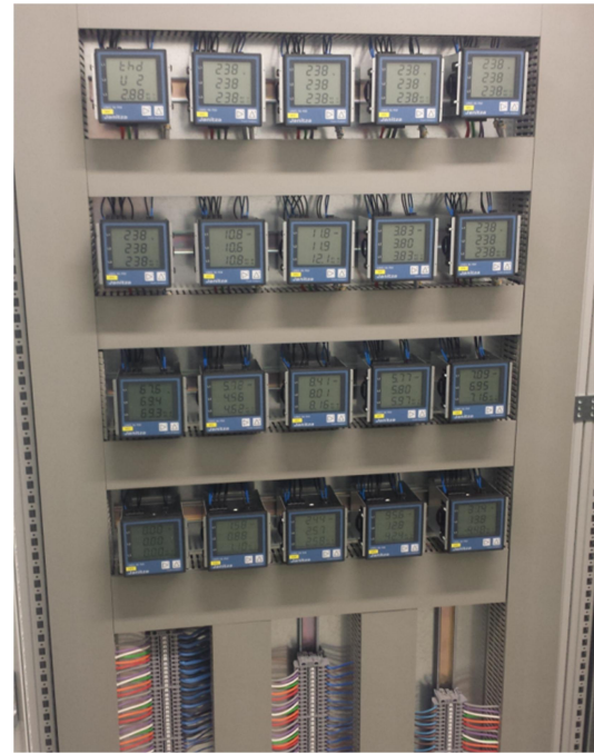
Figure 6.64: Installation of a set of electricity meters in a switchboard
