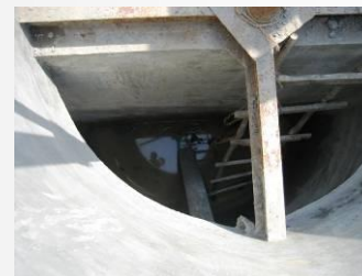
inlet chamber for toilet water
