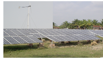
55 kW Solar and 3.5 kW Wind Electric Generator based hybrid system
