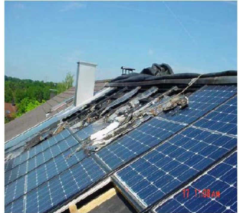
Module failure due to arching
