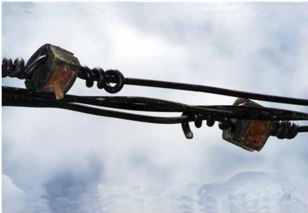
Good wiring connection
