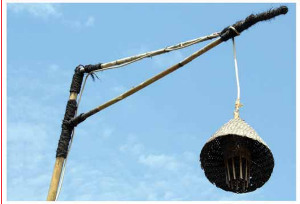
Bad example of a street light wiring
