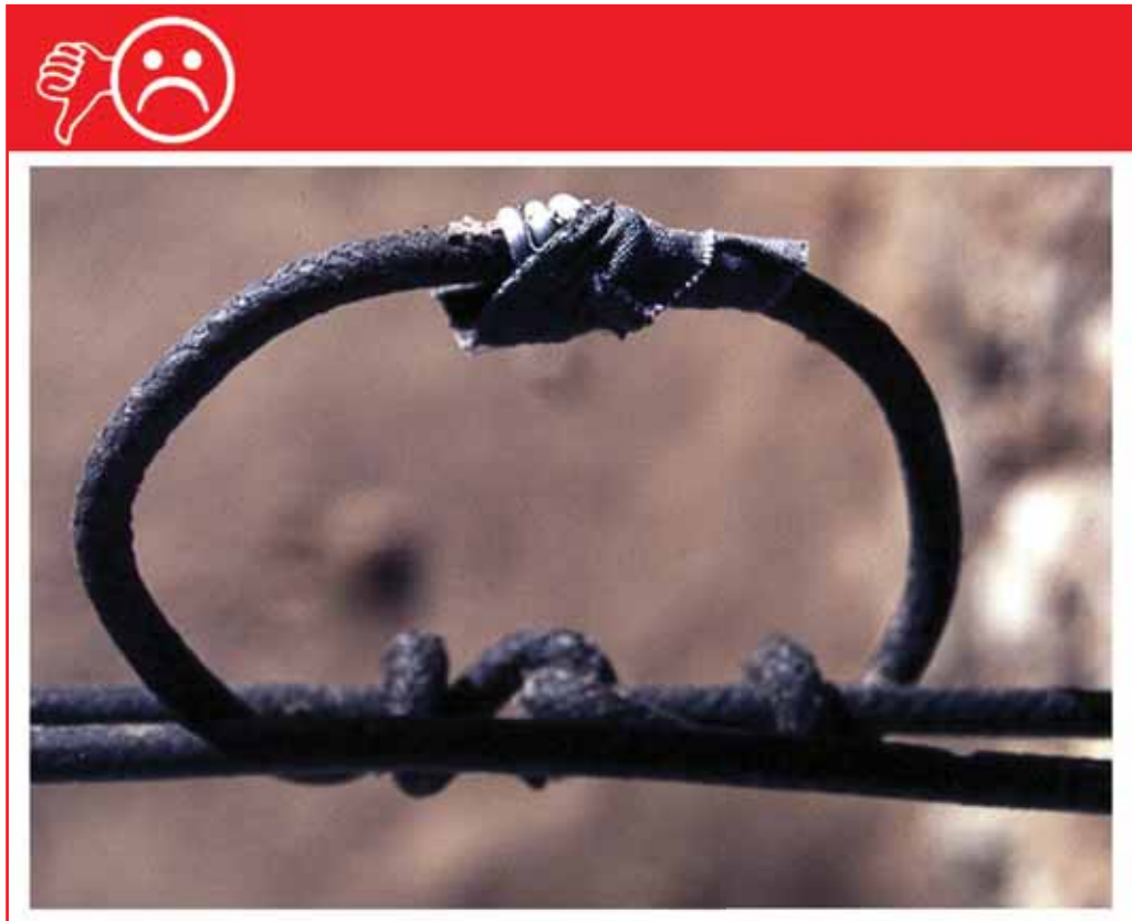
Bad wiring connection
