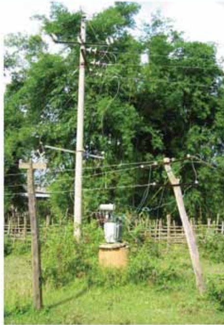
Bad example of distribution pole & lines
