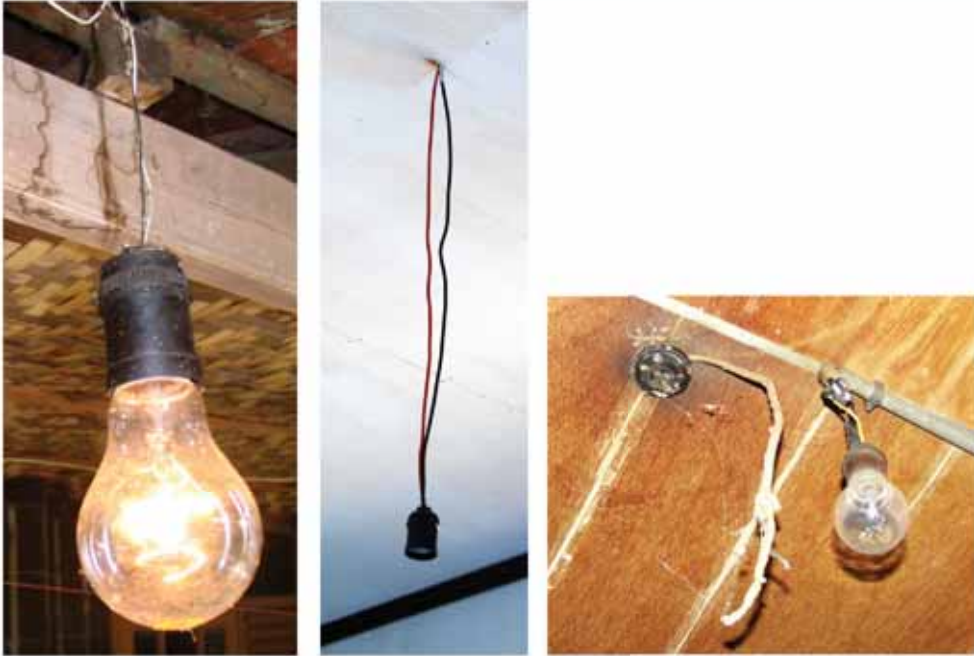
Lamp installations - bad
