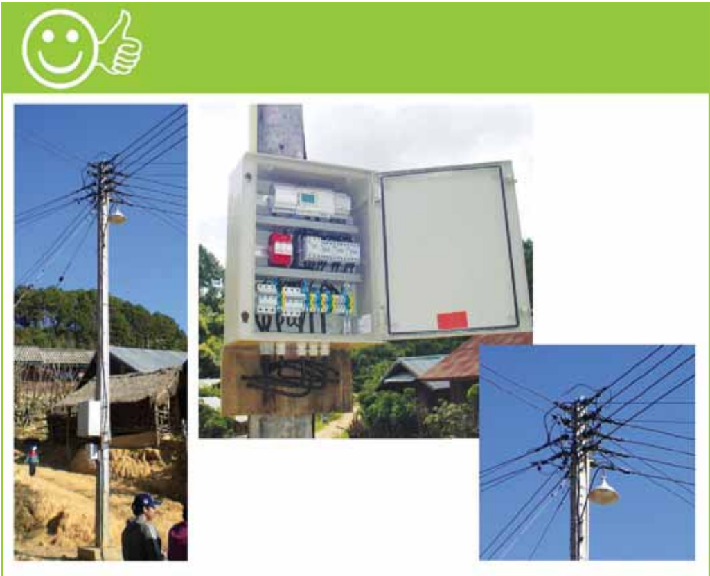
Good wiring connections
