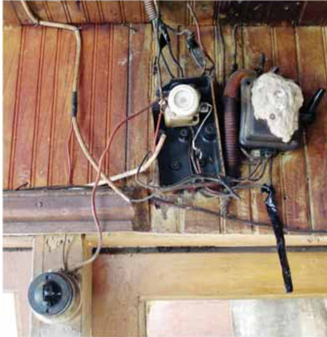
House wiring and fittings - bad
