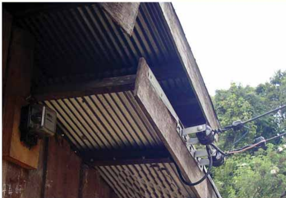
Service connection - good
