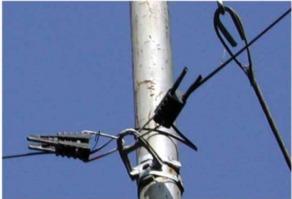
Good example of a wiring connection
