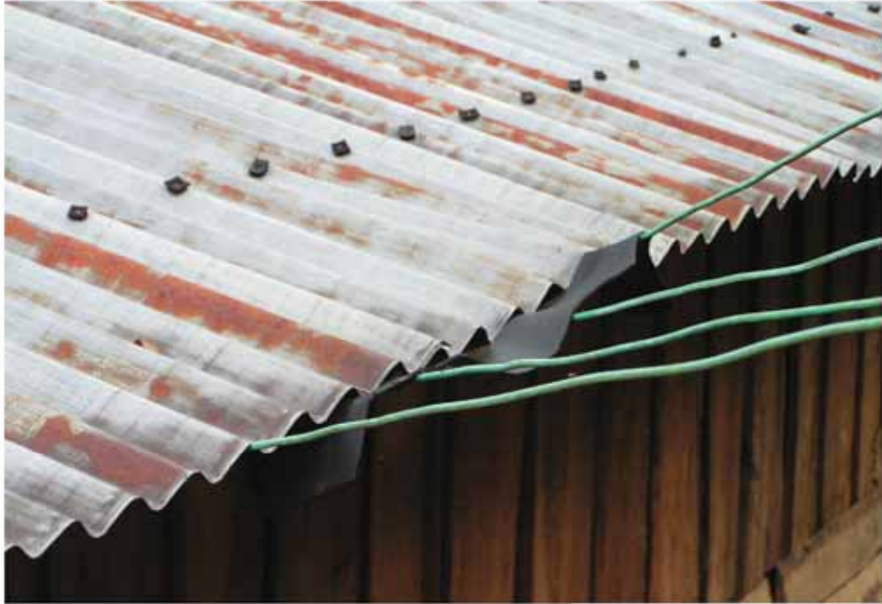
Service connection - bad
