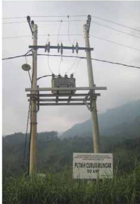
Good example of a transformer station
