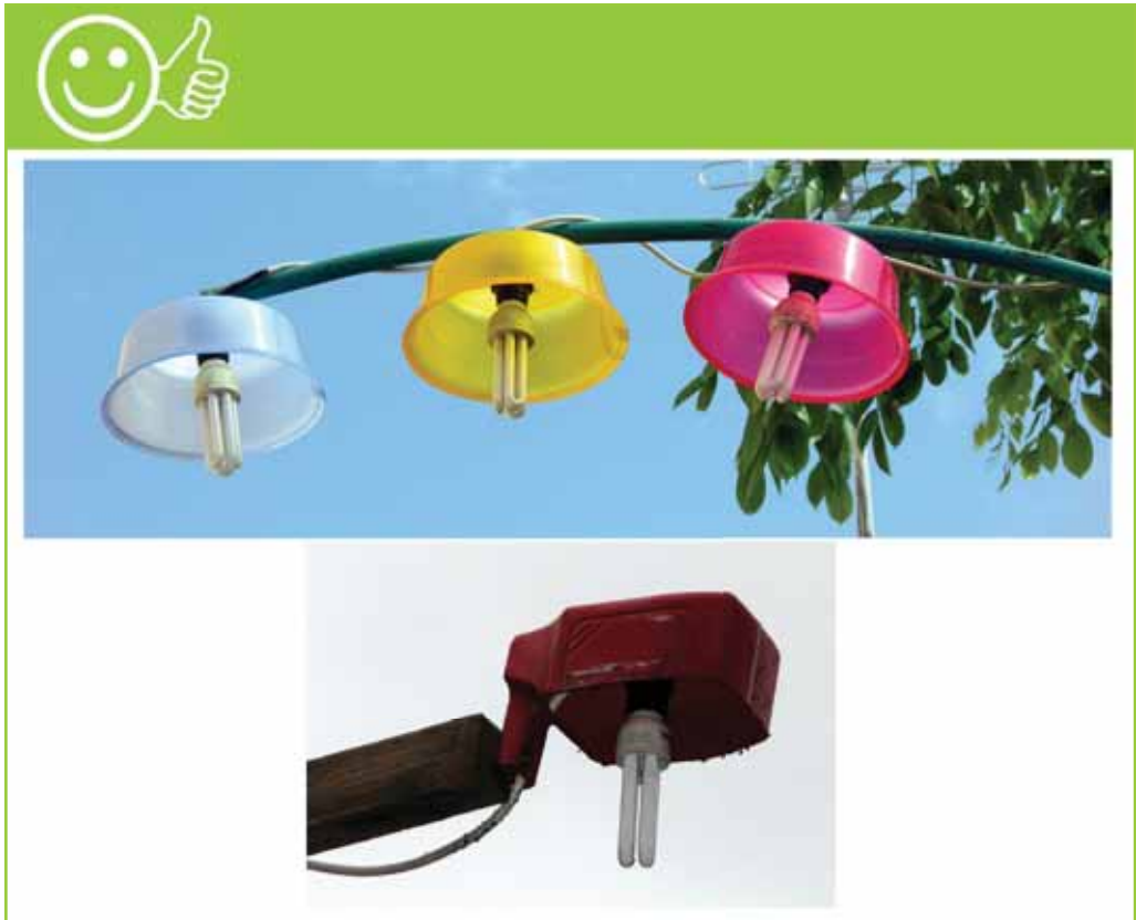
Good examples of street light installation
