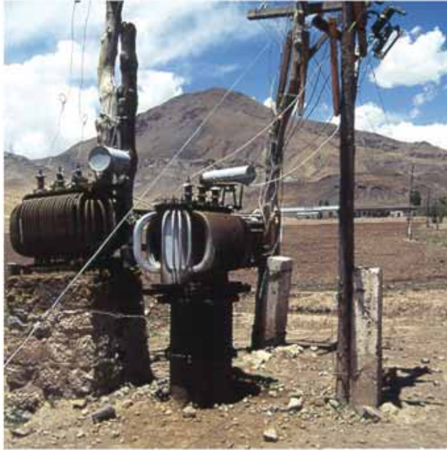
Bad example of a transformer station
