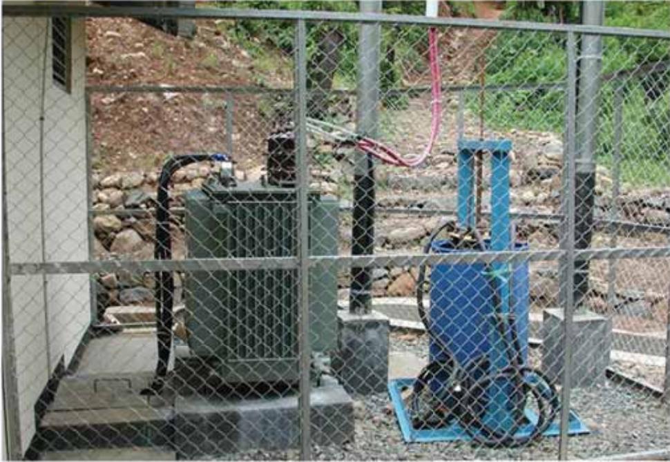
Good example of a transformer station
