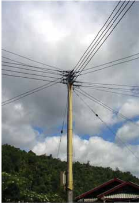
Good example of distribution pole & lines
