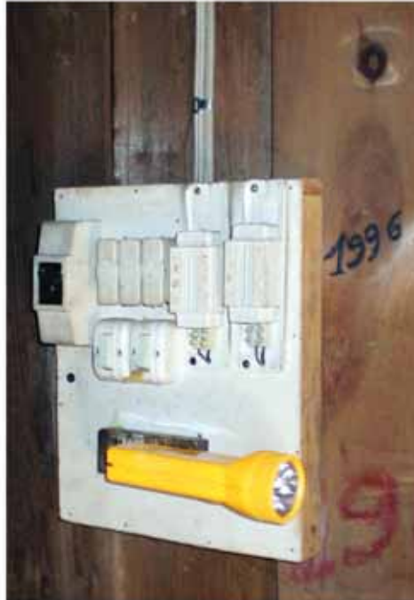
House wiring and fittings - good
