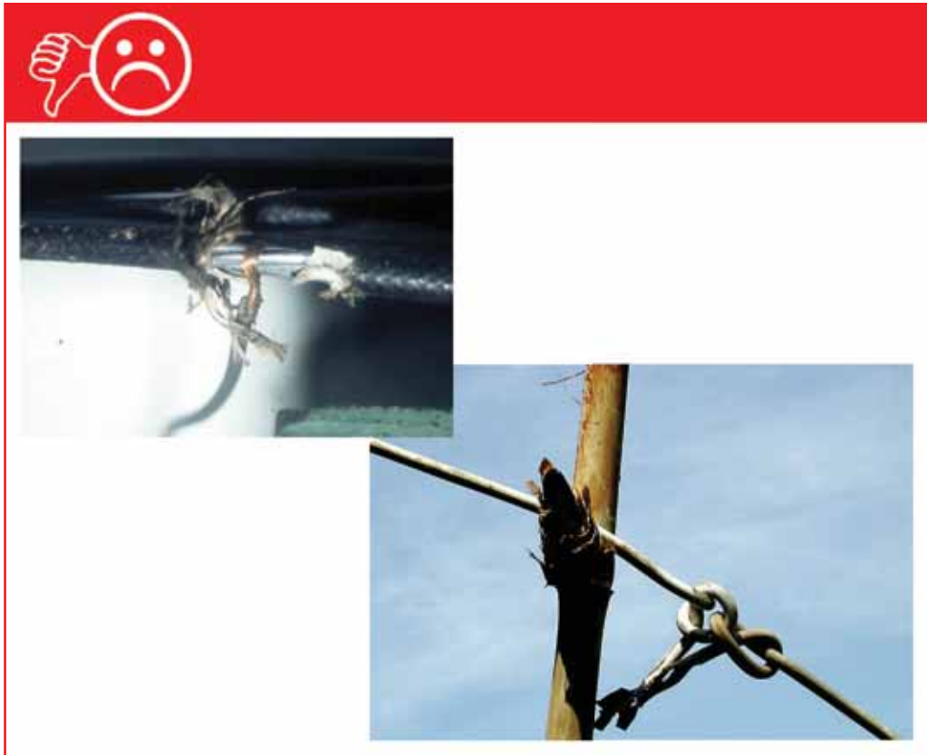
Bad wiring connection
