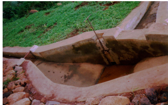
Figure 3.34: Desilting tank with flush out valve
