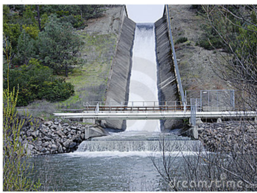
Figure 3.25: Chute spillway on a map (top) and at Napa dam, California (bottom)
