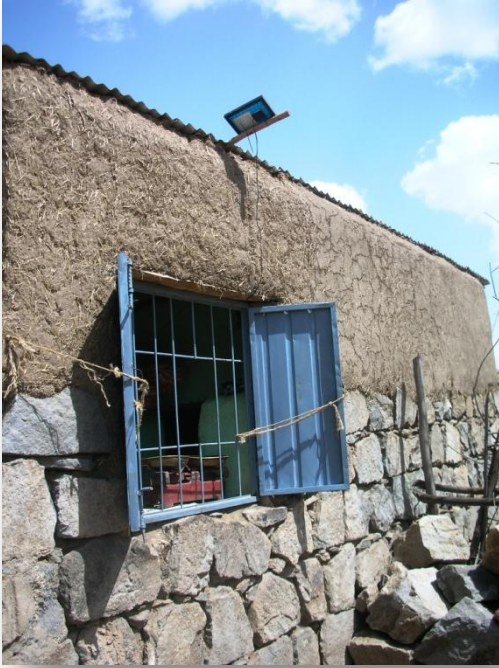
Shop in the village with a solar panel on its roof.
