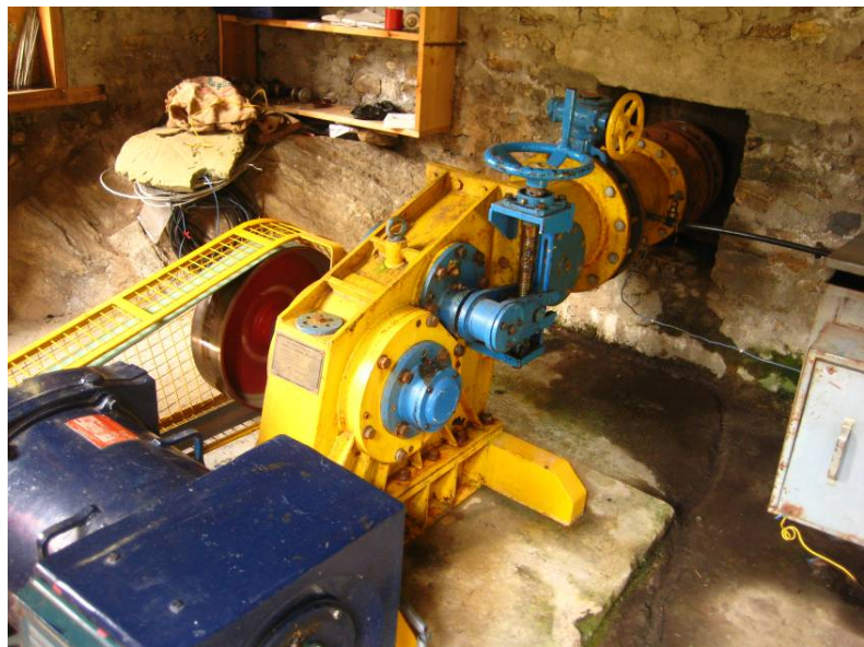
Turbine of the Basa Khola Micro Hydro Power Plant.
