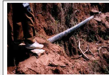
Figure 10-7 A length of pipe can be used to bridge a difficult gully with a small canal. The pipe is secured with rocks on either side.
