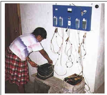
Figure 13-4 Battery charging with hydro power (Peru)
