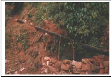
Figure 11-5 Pipe sections that span gaps must be supported at the correct height.
