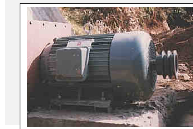
Figure 9-4 3-Phase Induction Motor (7.5 kW) with double-ended shaft, used as a generator. (Nepal)
