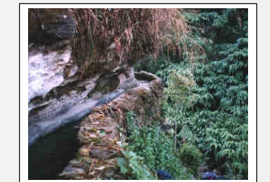
Figure 10-9 and Figure 10-10 show a raised canal that runs on a narrow ledge underneath a vertical rock face. The canal has a masonry lining and is supported by a high stone wall underneath.
