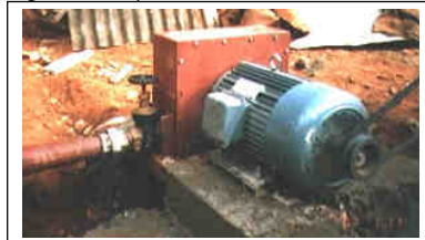
Figure 8-3 Installed Pico Power Pack
