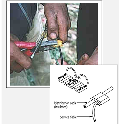
Figure 14-9 and Figure 14-10: Use of a tap splice to connect the service cable to an insulated distribution cable
