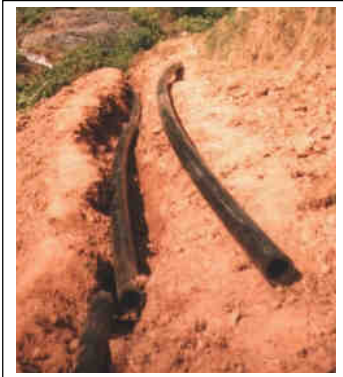
Figure 11-4 The penstock can be laid in a trench and then buried when the installation is complete to secure it
