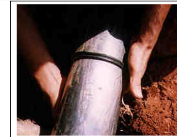
Figure 11-9 The plate is removed and the two sections are brought together forming a neat bead around the pipe.
