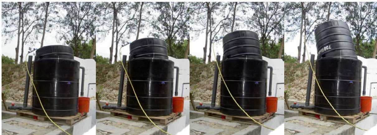
Figure 15: Continuous rising of gasholder proportional to gas production
