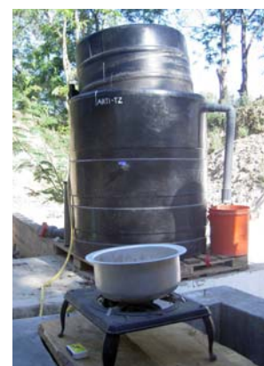
Figure 35: Gas stove attached on research CBS for burning tests
