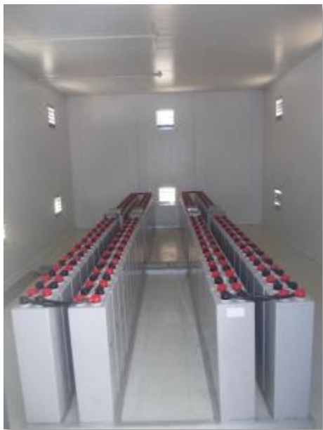
Main object (batteries) very well centred in the picture with correct orientation. Good lighting, sharp focus and picture shows other objects (ventilation openings, neat battery room, conduits).
