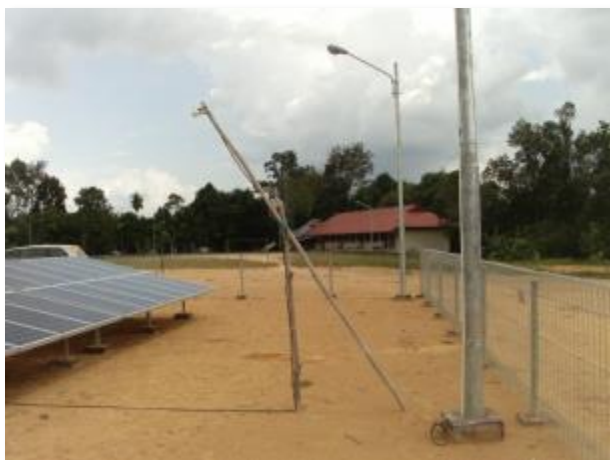
Very interesting picture showing a home-made streetlight, with a standard streetlight, BUT the car behind the solar panels is disturbing.
