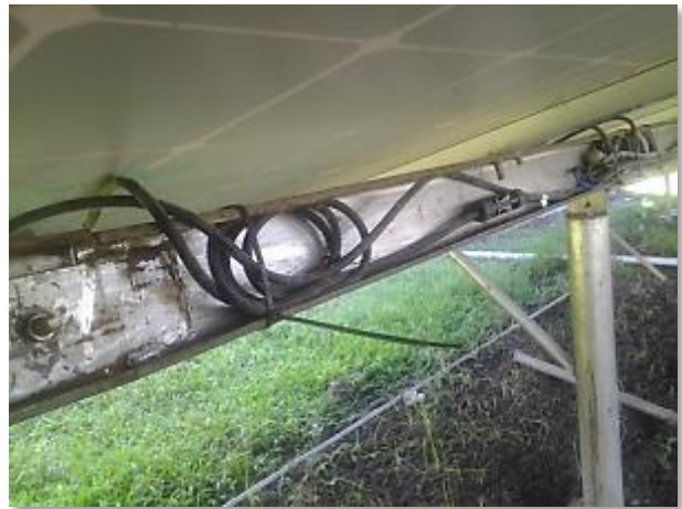
Picture with more than one “object” (in this case: poor wiring, corrosion on steel frame, no conduits and bolts not equal length) reveal more information.
