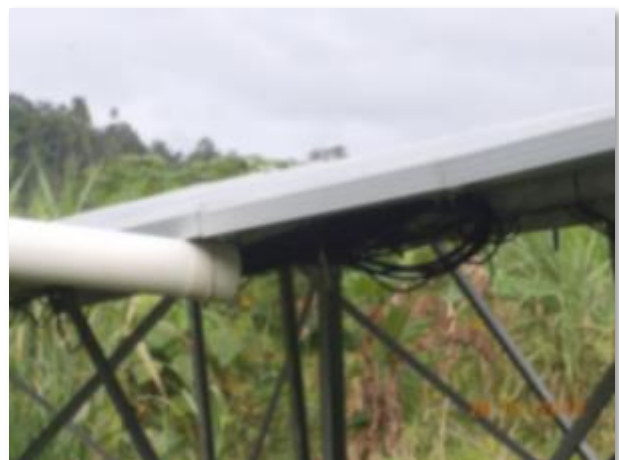
Picture out of focus, too low picture resolution (only 90KB), too close and wrong angle. Angle from below, taken from opposite direction (i.e. showing underside of panels and unsealed conduit opening) would have been better.
