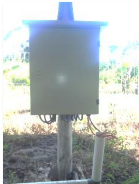
Picture with too much backlight and wrong orientation (landscape orientation from slightly greater distance would show ground conduits and avoid backlight).
